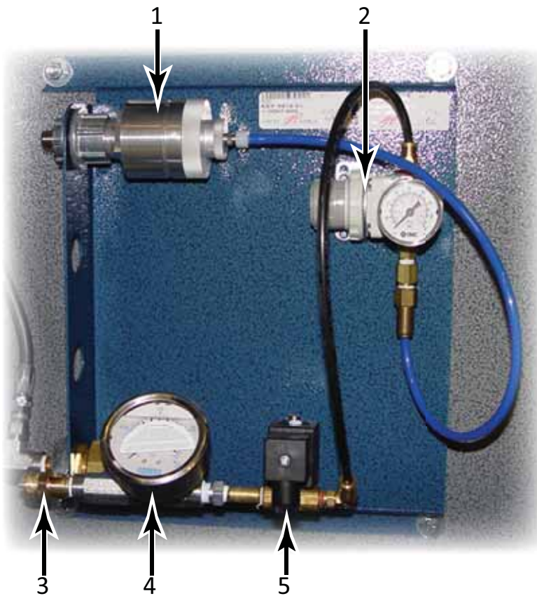
Figure 8-3 Regulator and Monitors
